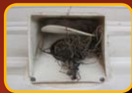
Bird nests are a major cause of vent blockages.
